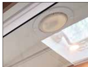
Ventilator i brusebad (TDL, 780 DGLE)
